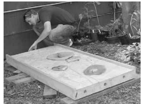
Installer Matt Tong looks at the MsK Memorial Wall to prepare for its installation near the greenhouse.
